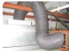
Energy-Saving Duct for the Firing Furnace
