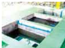
Ferrite sludge waste water treatment system
